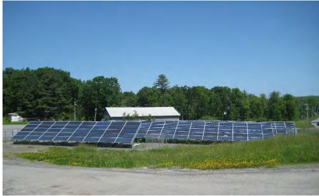
3.13. Solar Panels at Town Highway Department
